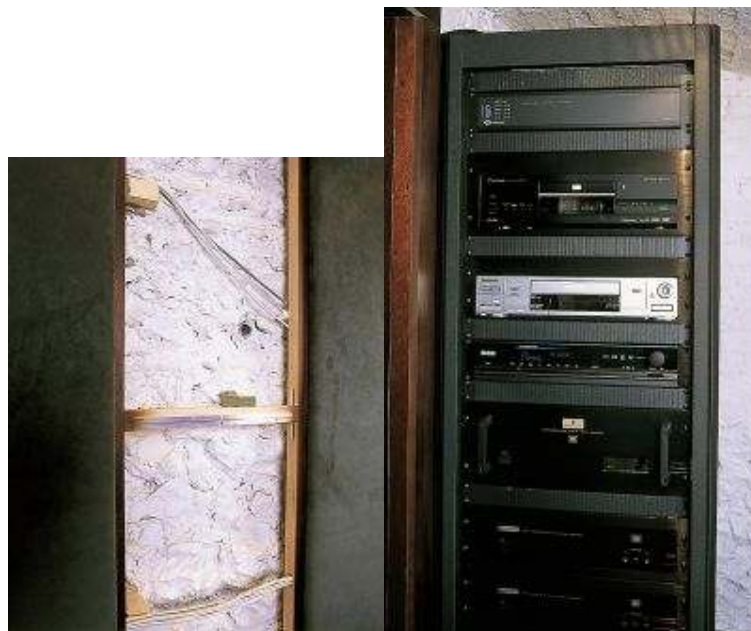
Chic fabric-covered walls conceal the necessary metres of cabling and pipework
